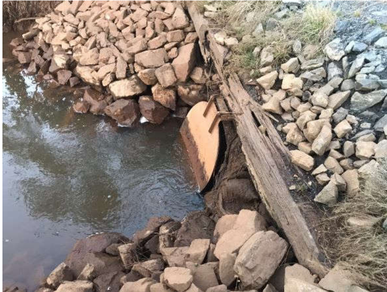
Photo 6.1: Tidal gate located on Green Meadows Road
